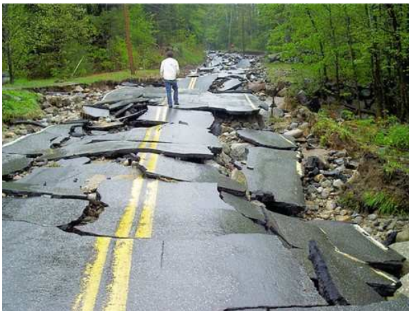
Figure: Road Damaged after Flooding, Source: AccuWeather.com
