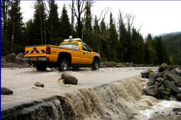
Figure: Roads are Damaged by Floods, Source: The Oregonian
